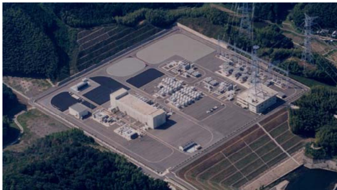
Kii Channel HVDC Transmission - 2000
