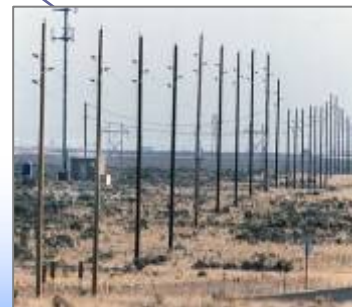
Power Grid Test Bed
