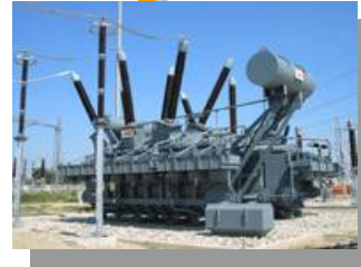
Phase Shifting Transformers
