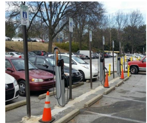
Level II Charger
