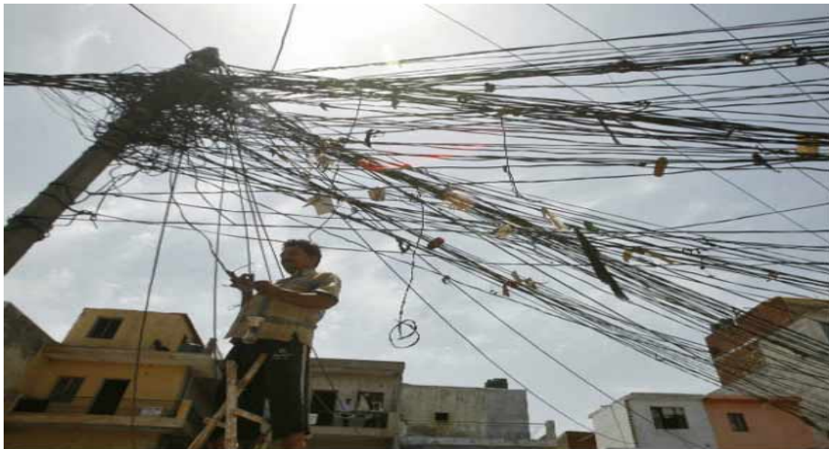
A man stands on a stepladder to fix tangled overhead electric power cables at a residential area in Noida, India, June 1, 2011 (Parivartan Sharma/Courtesy Reuters).
