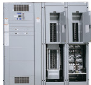
Integrated Facility Systems
