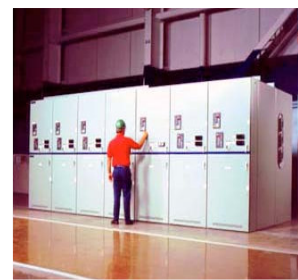
Motor Control & Switch Gear
